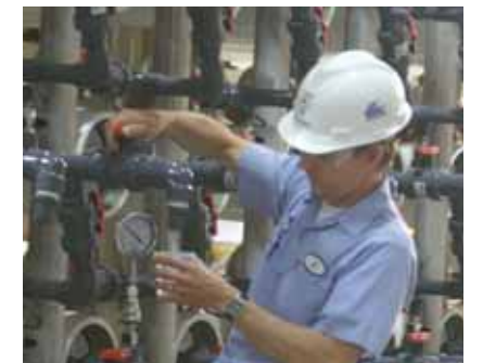
Reverse osmosis system at the Bingham Canyon Water Treatment Plant
