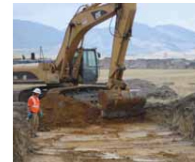
Bingham-Magna Ditch during cleanup
